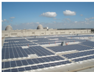
Solar Panels on the OCCC's North/South Building rooftop
